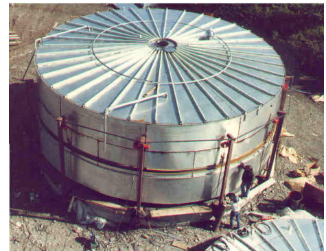
With second course welded underneath the first, tank is lifted into the air to add the third course.
