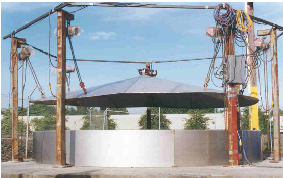
Cone is fabricated and lifted five feet in the air. Then, the first course is welded to the top.
